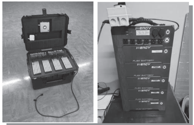
SmartBox and Solar Power system installed in the village of Empash
